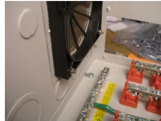
E-Panel earth ground bus (AC & DC)
