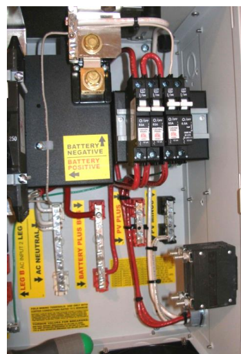
63 amp din rail DC-GFP wired with a 63 amp PV disconnect and a 63 amp controller output breaker.
