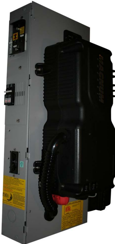
E-PANEL FOR MAGNUM MM SERIES AS INSTALLED
