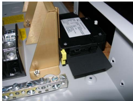
Supplied insulators to achieve required separation of AC and DC circuits
