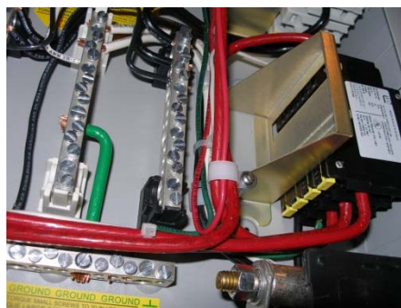
Ground to Neutral connection
