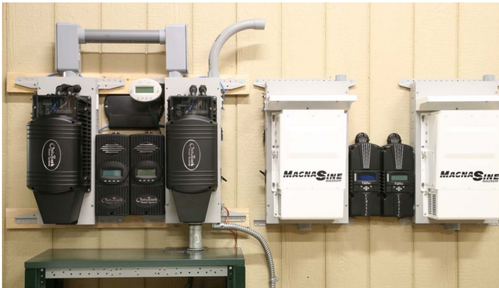
OutBack and Magnum horizontal stacked systems
